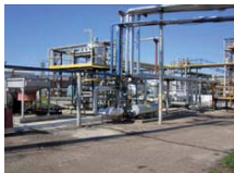
Fig. 2: Industrial installation for direct selective oxidation of H 2 S
